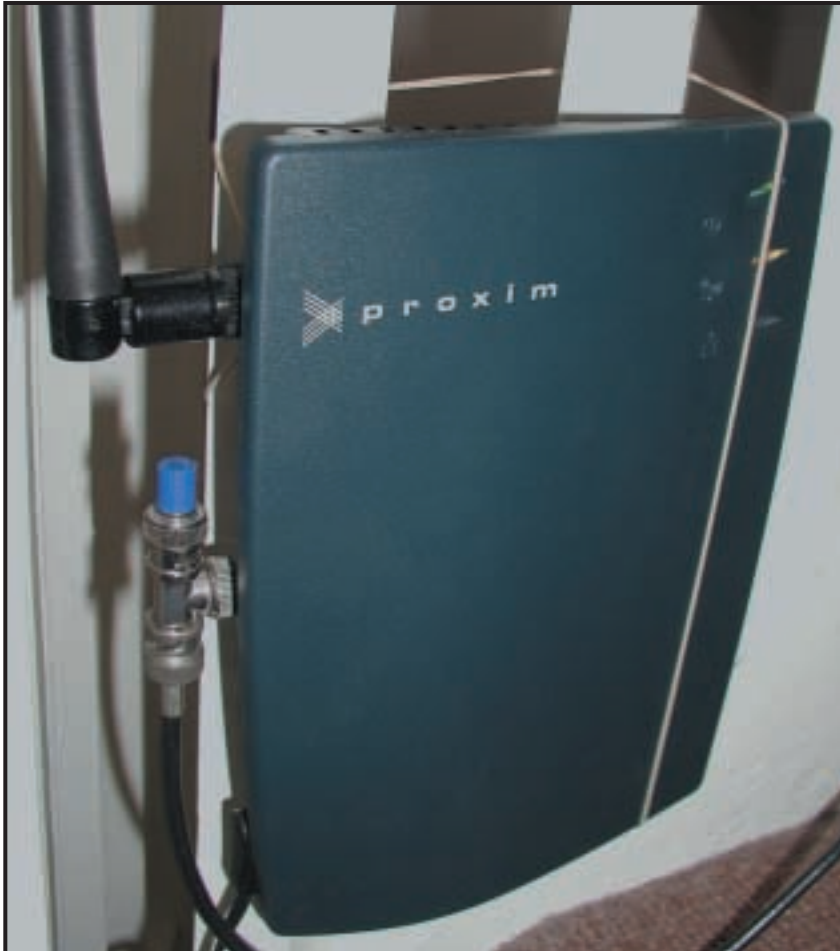
The RangeLan2 Access point is light enough to attach to the bannisters of the Bidmead staircase with a single elastic band. Photo courtesy of Dave Williams
